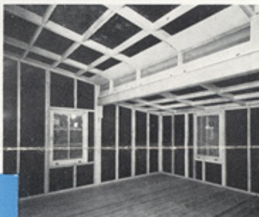
Photo of interior showing 15 ft. screened and shuttered ventilator, and 6 x 8 inch beam supporting roof.
