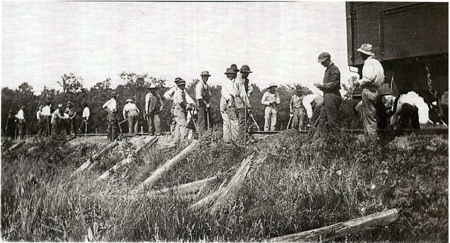
Photo #10: Pictured here are at least 25 men involved in setting ties and rails. The broken and split ties are off to the side as the work progresses. By evening the track was repaired. The newspapers reported trains ran on schedule on Friday the next day after the accident.
