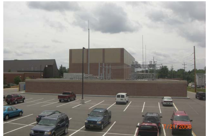
Satellite Energy Facility
